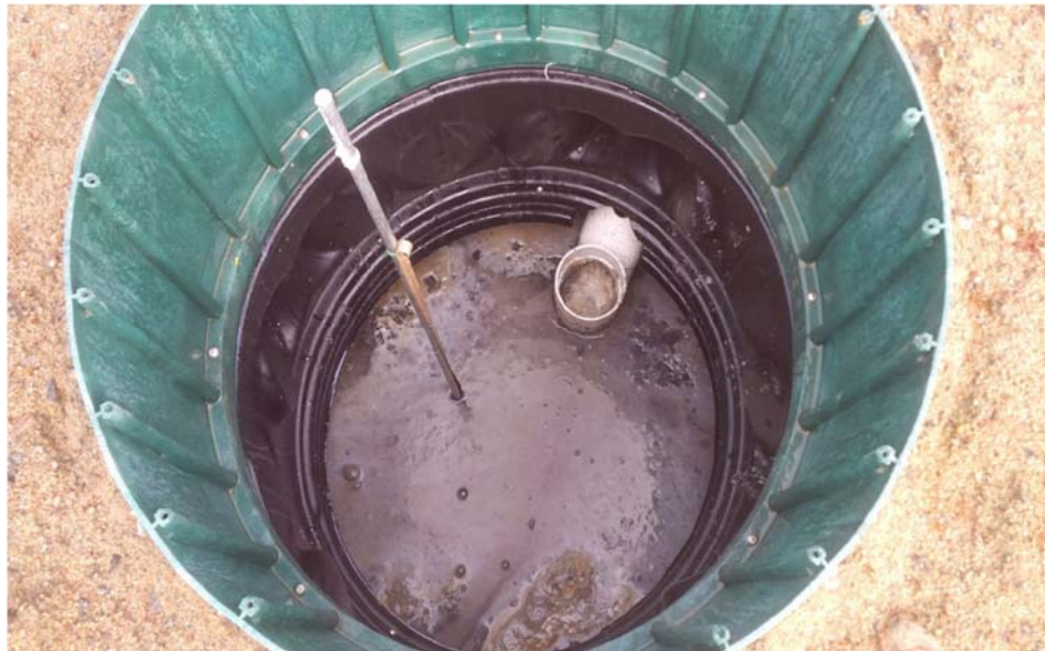
Figure 4a. After 8 months of BNQ testing, the septic tank is completely full of solids.
