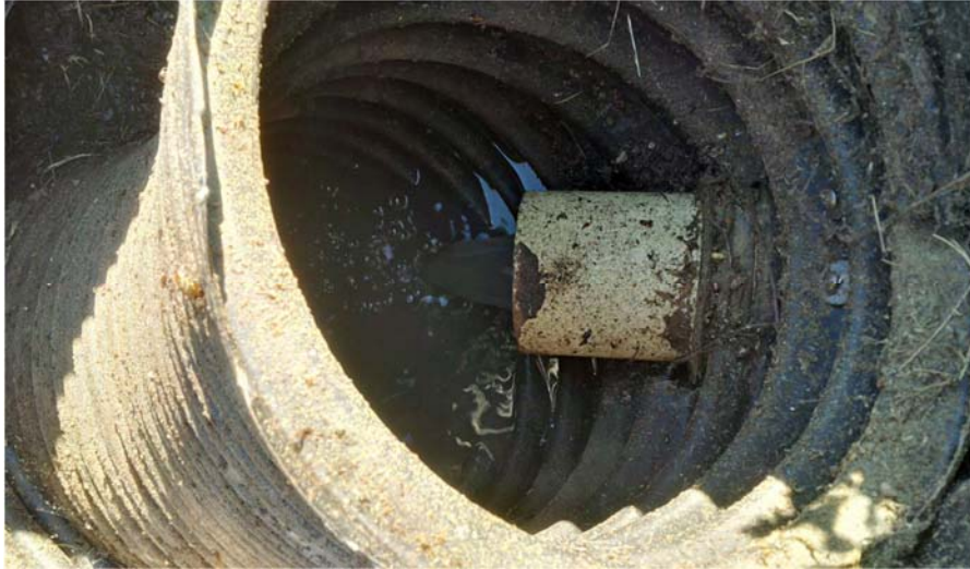
Figure 6. Raw sewage is directed through the InnerTube pipe before entering the greater tank volume.
