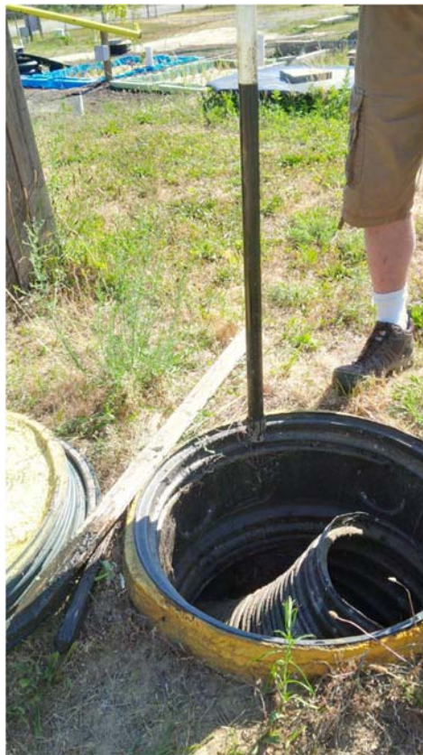
Figure 7. After 3.5 years of continuous dosing scum and sludge have accumulated at the tank inlet.
