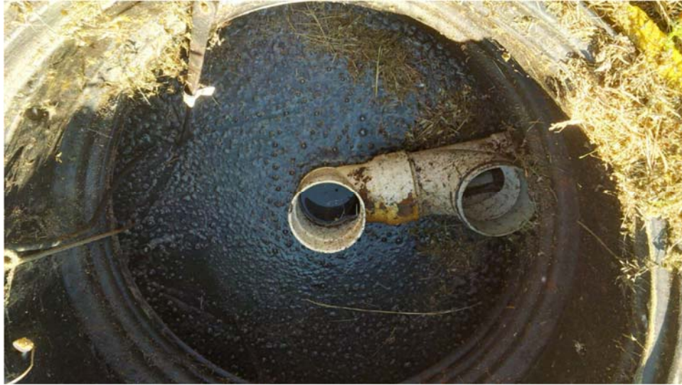
Figure 8. After 3.5 years of continuous dosing no scum has formed at the tank outlet and sludge depth is 6”.
